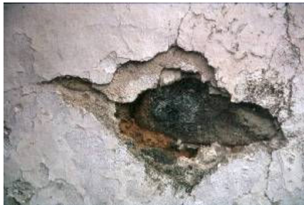
Figure 2. Loose of adhesion of renders at Sta. M a de Penamaior due to cement-based mortars.
