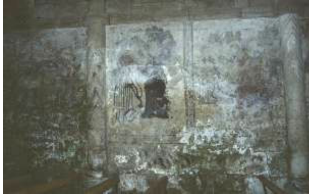
Figure 4. Interior condition of St. Xiao de Moraine due to the used of cement mortars in the outside: biological deterioration of mural paintings and soluble salt deposits.
