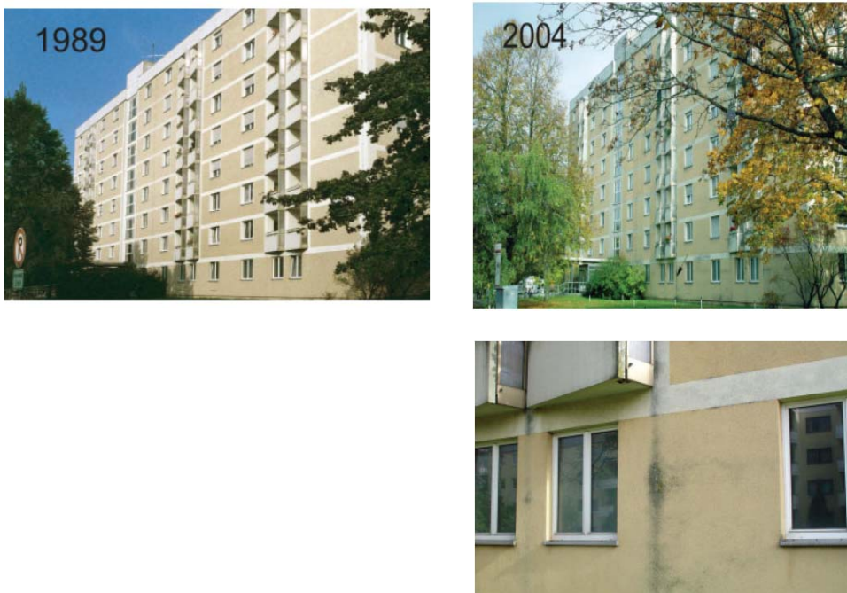
Figure 5: View of the west facade of a renovated building with ETICS in Munich in 1989 (top), three years after refurbishment, and in 2004 (below) with the growth of algae (arrow below)
