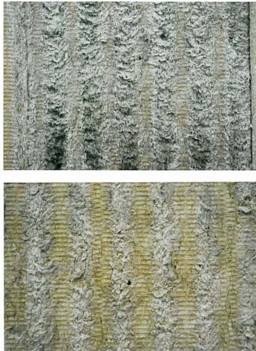
Figure 1: Surfaces of stone-wool fibre slabs after 4 years of weathering in western orientation with driving rain load (top) and east (bottom)
