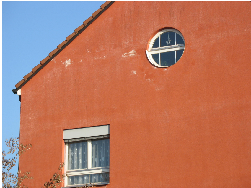
Figure 1 - Cementitious render with efflorescence. (Photographed by J. Lang; Elotex)
